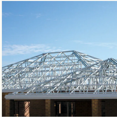
SCG Roof TRUSS
